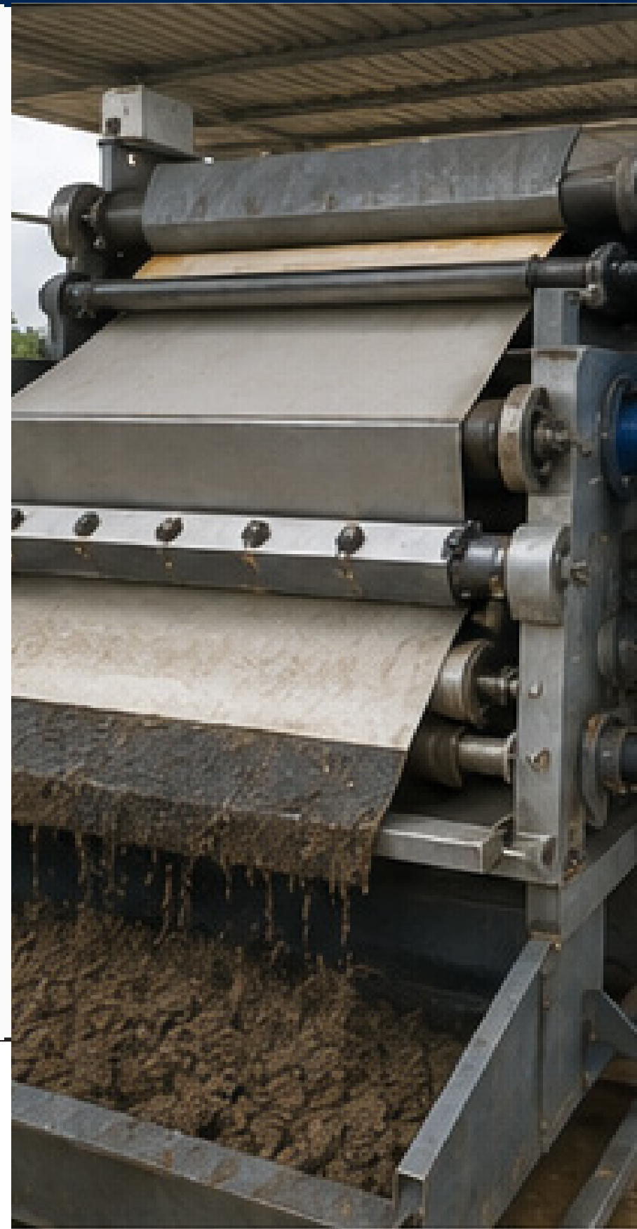
Sludge Dewatering System
